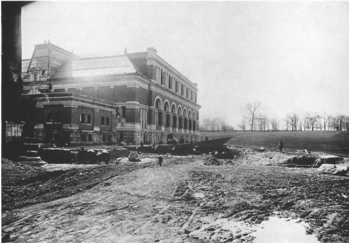
34. Weston and Tuckerman's north wing from Fifth Avenue (with the boiler house in the foreground). Photograph taken April 24, 1906, during excavations for the first McKim, Mead and White wing
